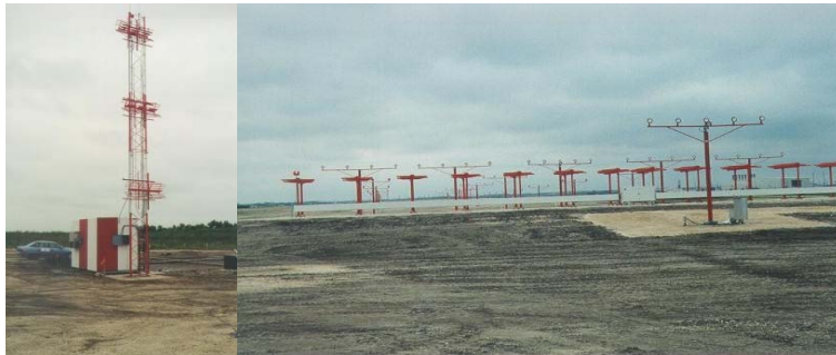
Instrument Landing System
